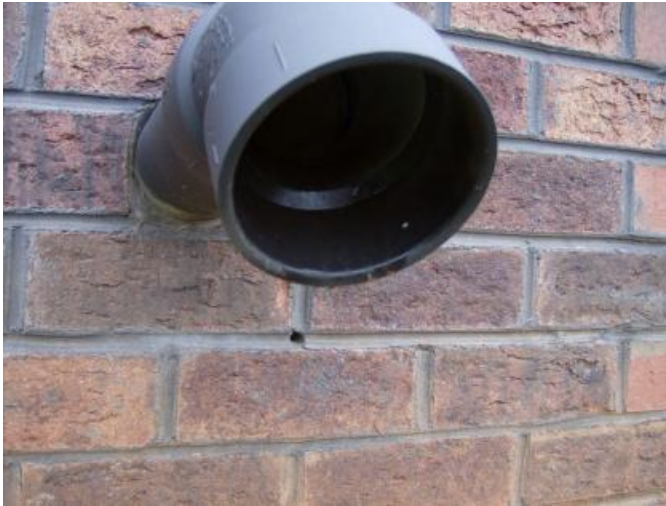
View of flue pipe missing the entrance screen
