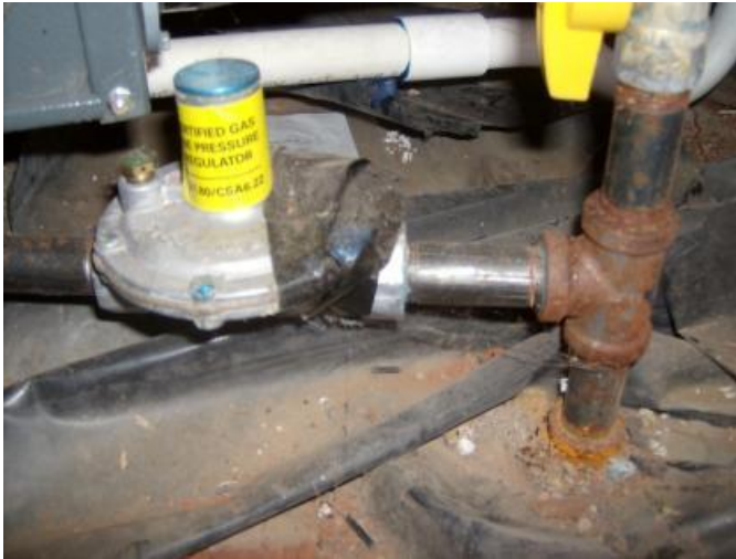
View of gas regulator at the crawl space furnace.
