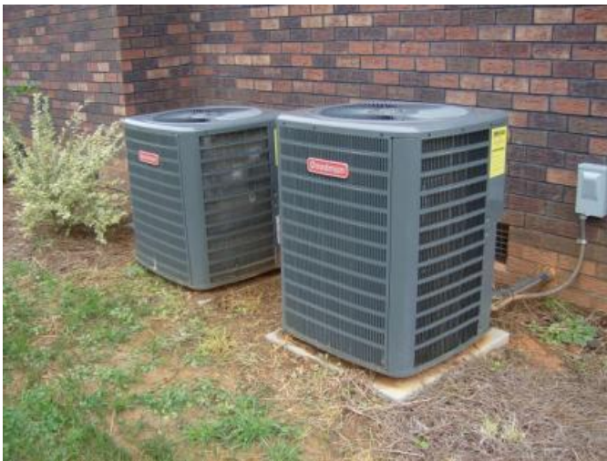
View of AC units
